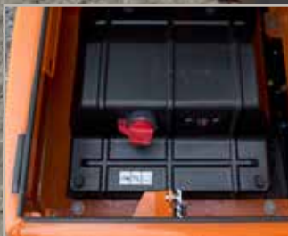
Battery cut-off switch
